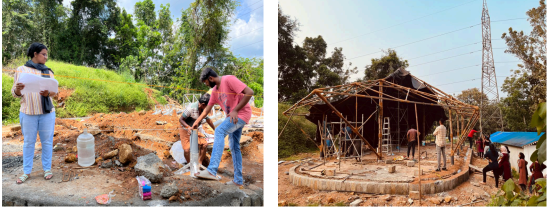
Figure 2, 3: Students work on a pavilion as a part of a DesignBuild exercise at SEED, Kerala.
