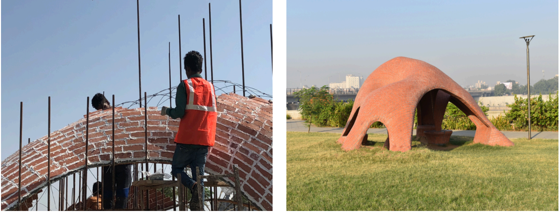
Figure 6, 7: The Digital Craft Pavilion – a student DesignBuild project by CEPT University in collaboration with artisans from Hunnarshala.
