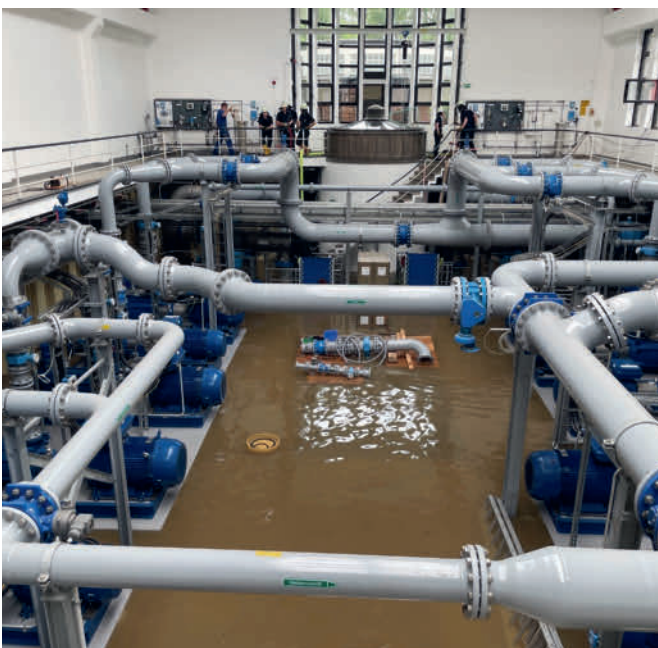
Bild 17.5: Wassereintritt in das Pumpwerk des Wasserwerks Essen-Kettwig (RWW) Fig. 17.5: Inlet of water into the pumping station of the waterworks Essen-Kettwig (RWW)
