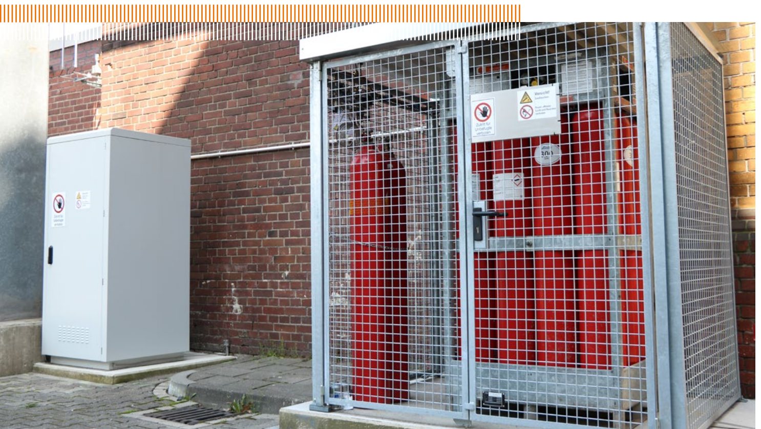
Emergency power supply system operated by Netzgesellschaft Düsseldorf at its Flिंगern site
