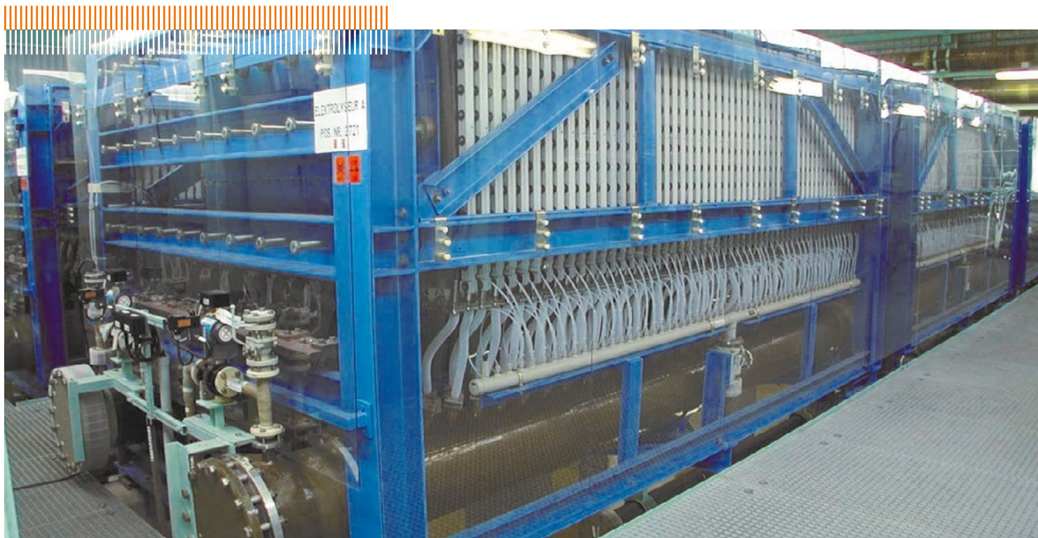
Chlorine-alkali electrolysis in Hürth-Knapsack: 310,000 t of chlorine per year, 203,000 Nm 3 of hydrogen per day
