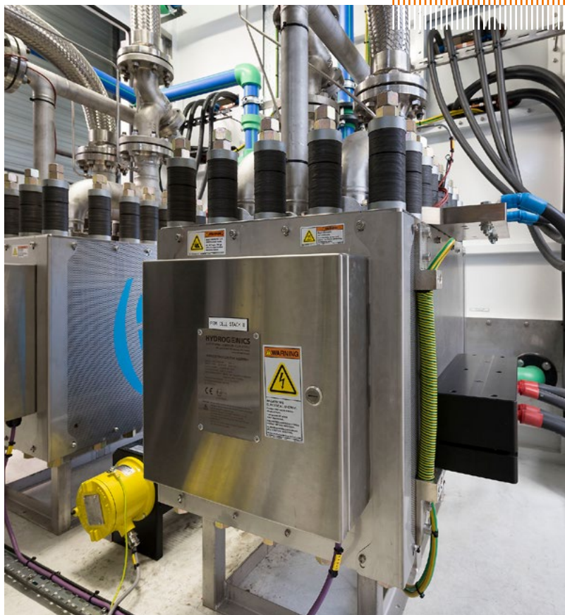
Hydrogenics PEM Electrolyzer (HyLYZER®-230-30), 230 Nm 3 /h (1.2 MW)
