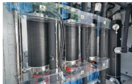
In Ibbenbüren RWE operates a Power-to-Gas project and is researching an innovative electrolysis process.
