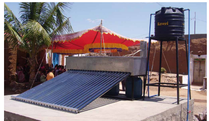
Solar-thermal desalination plant
