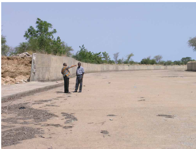
Tono irrigation project, Ghana
