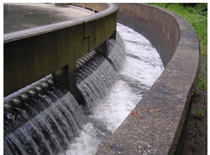
Stormwater tanks are used to treat stormwater in combined or separate sewerage systems and in road drainage. MUAS (2)
