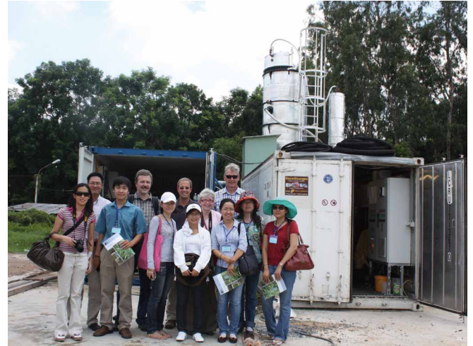
A partial view of the pilot plant with some of the project partners and a group of Vietnamese visitors. Prof. Dr.-Ing. J. Fettig
