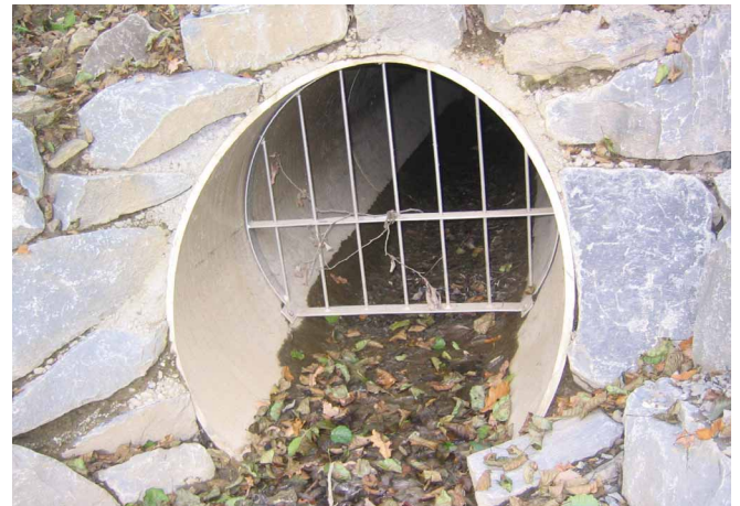
Exit of the sewerage system
