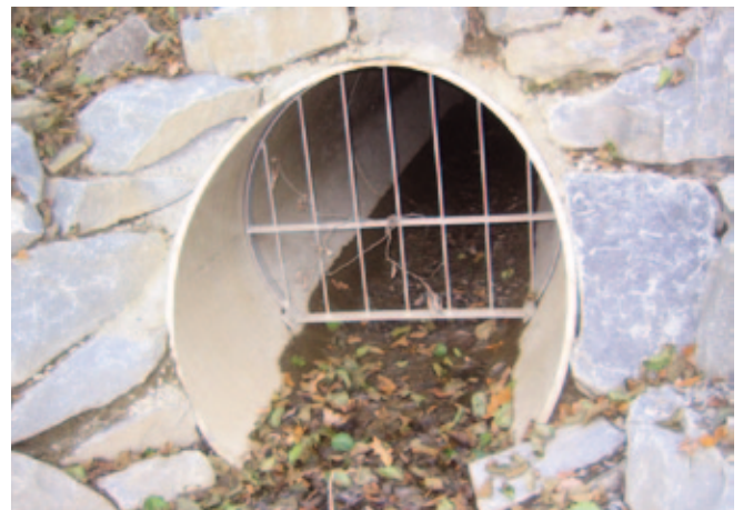
Exit of the sewerage system
