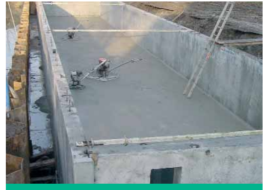
Filterbasin, which cleans the first most polluted part of sewer water when an outlet occurs.
