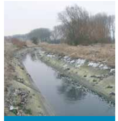
Concrete banks of the Espierre have to be restored for more ecological quality.
