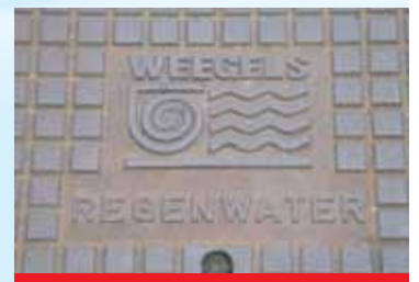
Often the change from a combined sewer system to a separate one for waste water and rain water is costly – but worth it.
